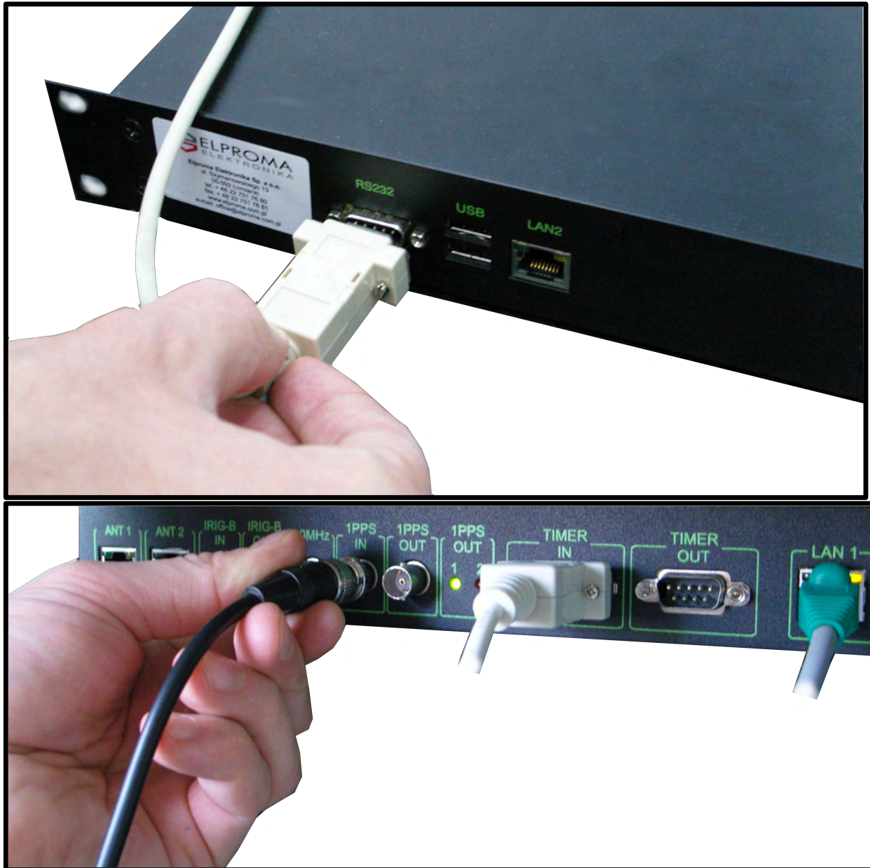
Connecting PPS (BNC) and ToD RS232 cables to NTS (the NTS-x000 back panel view)
