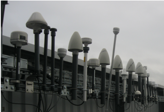
Figure 30 The example of a faulty installation: the receivers installed too close one to another, disturb one another and are connected to the lightning installations. Photo provided by Chronos (UK) and presented during IFTS 2016 Prague meeting.
