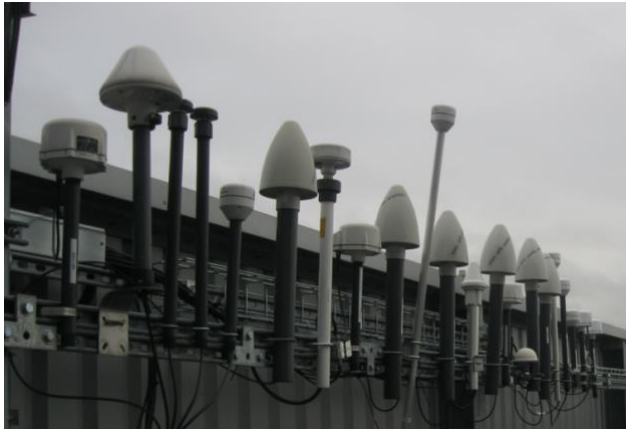
Figure 30 The example of a faulty installation: the receivers installed too close one to another, disturb one another and are connected to the lightning installations. Photo provided by Chronos (UK) and presented during IFTS 2016 Prague meeting.
